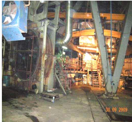
Figure 1. Ventilation mill in Kostolac B thermo power plant
